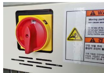
► Fig[7-16] – power on status
